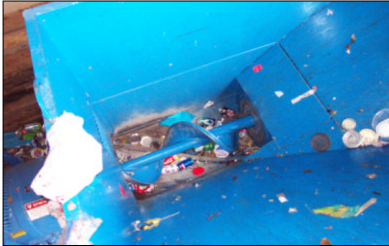
3) Overhead view into hopper showing auger mechanism
